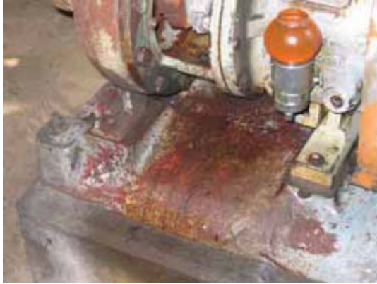
Fig 2.3 - Bearing lubricant leakage from an unbalanced lubricator.
