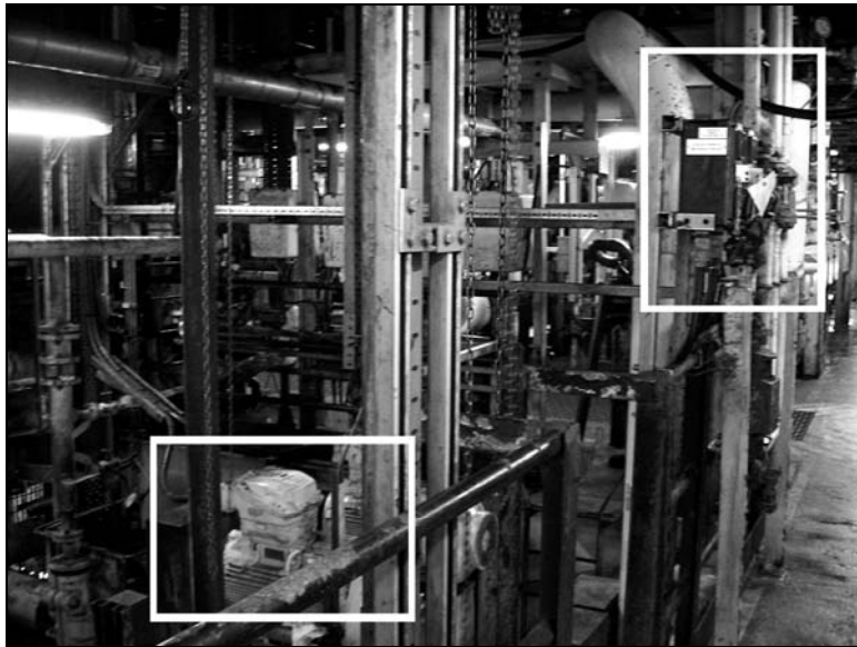
Fig. 17 - View of the application showing the pump bottom left and the reservoir top right.
