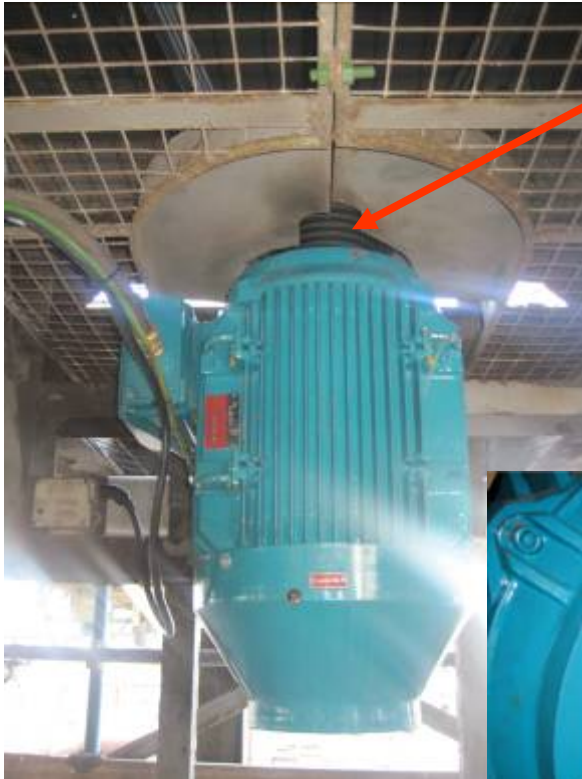
LabTecta TE installed
